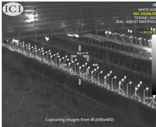
Pilot Inspection on a Petrochemical Ground Flare (Taken from a UAV with an ICI 9640P via the Sensor Control Module)
